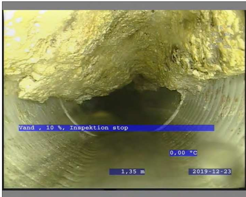
Foto: 5_4A, Medie #: TV2-414, 00:00:29 1,3m, Vand , 10 % / Inspektion stop
