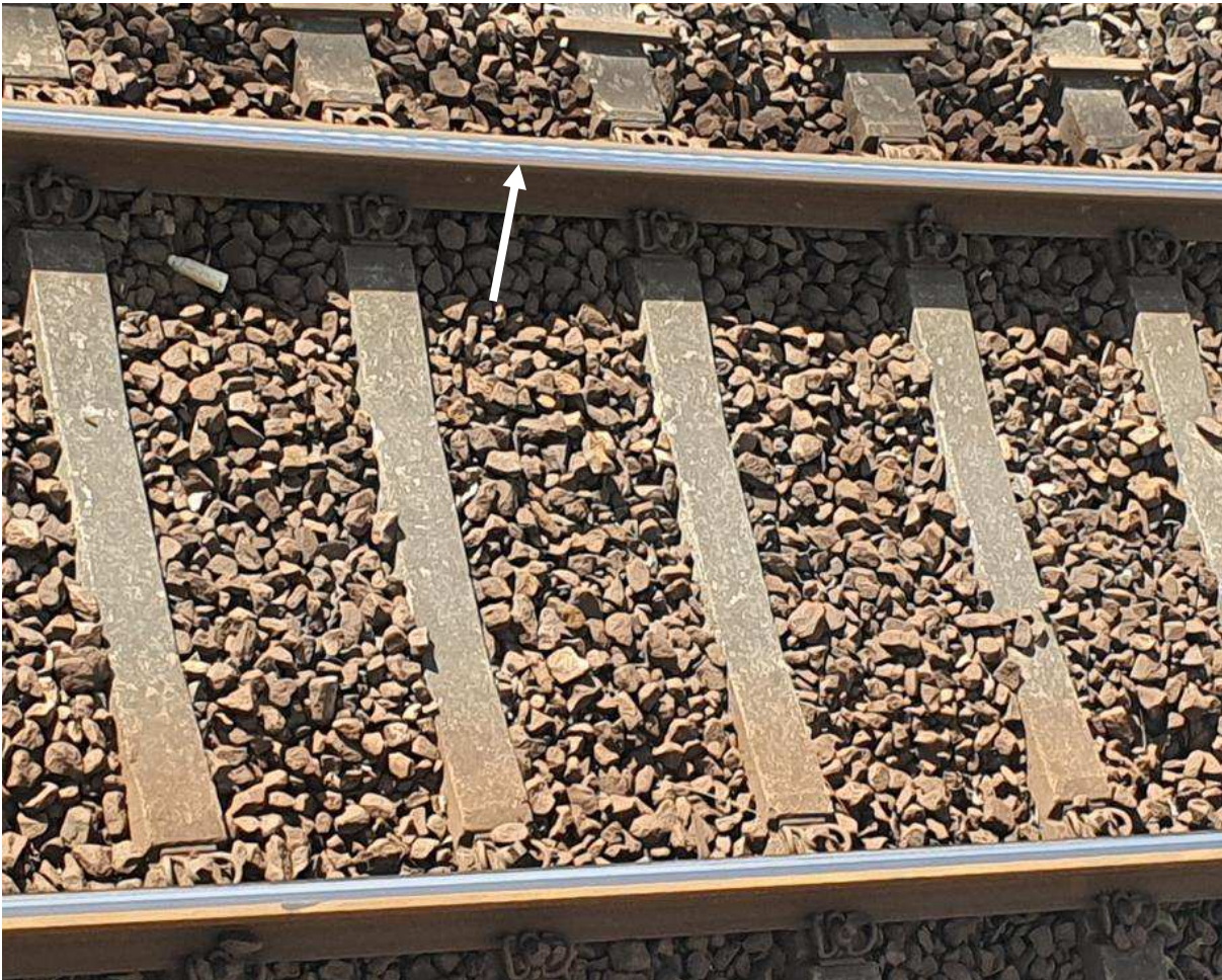
Figure 4 – Corrugation on the rail head of the inner rail in the northbound track because of stick-slip behavior
