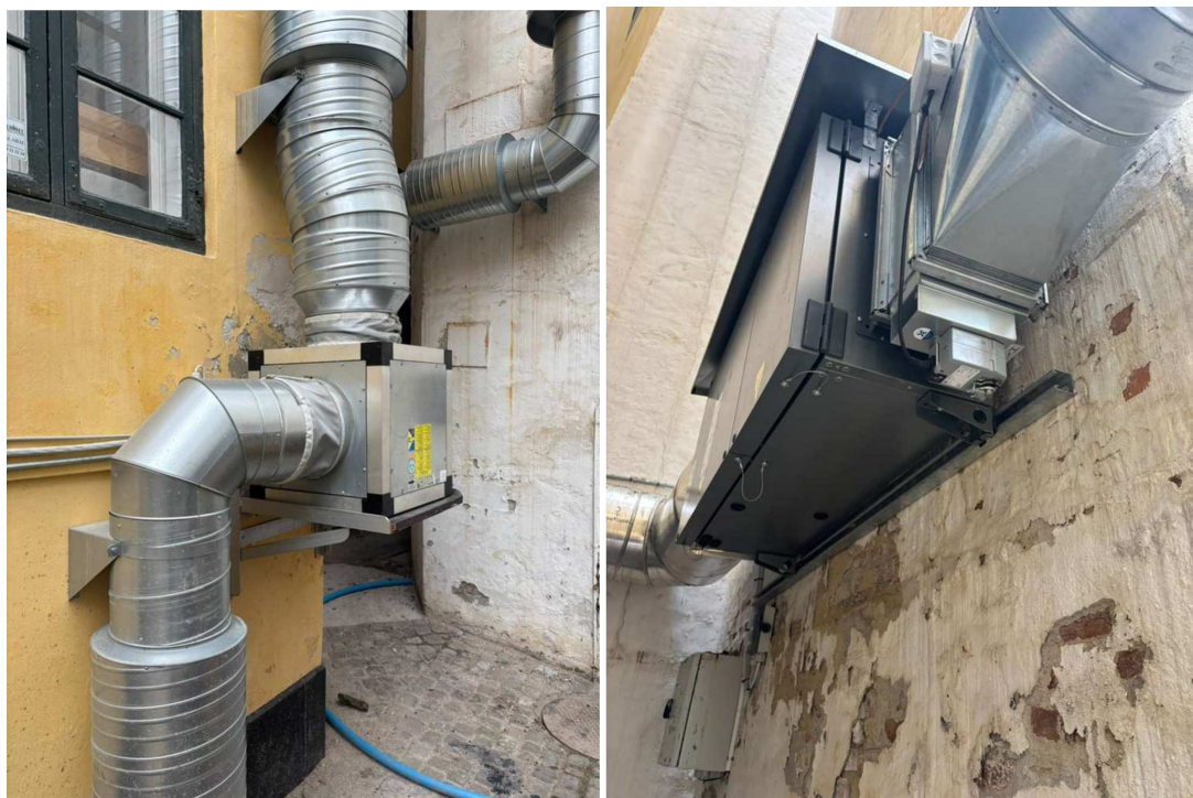
Figure 17: The cooling and ventilation system whose noise was measured at the Miljøpunkt Indre By & Christianshavn's office
