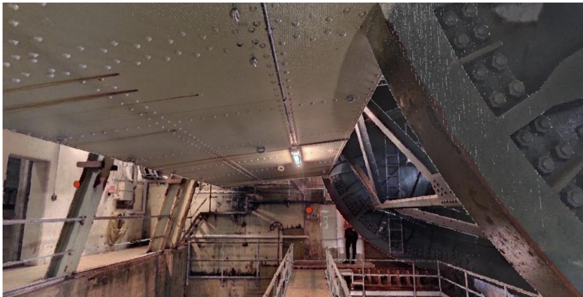
Figure 6 Photo, underside of the fixed counterweight. The rows of rivets lengthwise and crosswise show the location of internal steel bulkheads.
